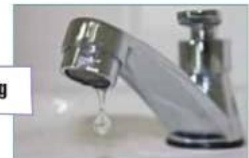
tap is leaking
